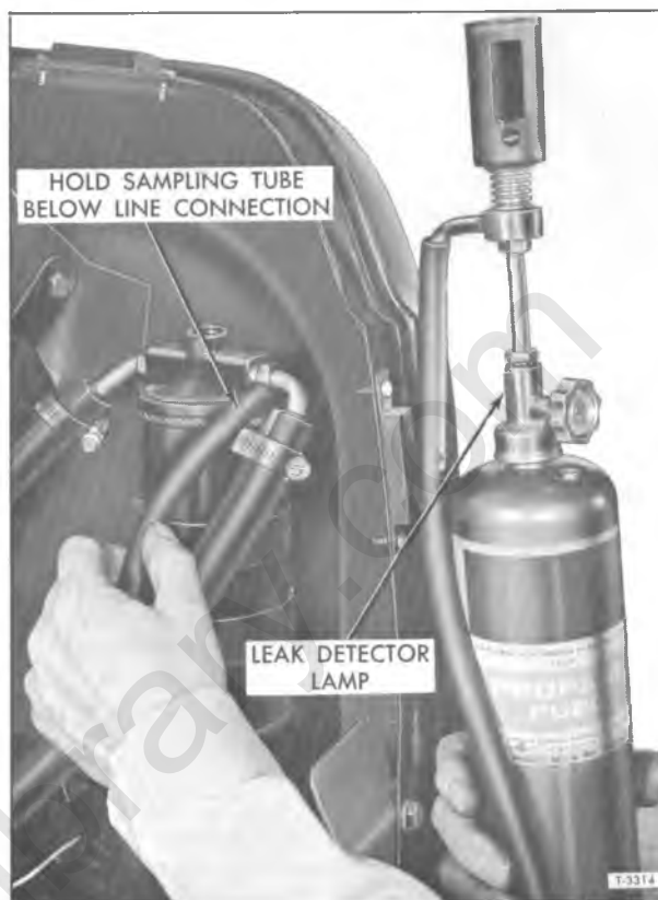
Figure 13—Checking for Refrigerant Leak
